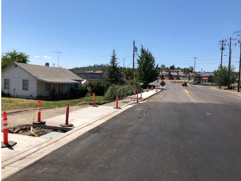
The last power pole on the south side of Linn Road was removed by Pacific Power.
