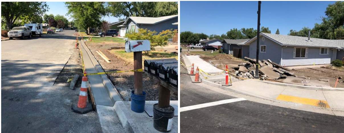
Work on side streets for new driveways and property owner modifications continued.
